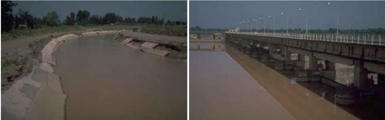
Fig. 9 : Damage of lining of downstream irrigation canal (left) and several counter weights for gate lifting of diversion structure of irrigation scheme were falling down (right)
