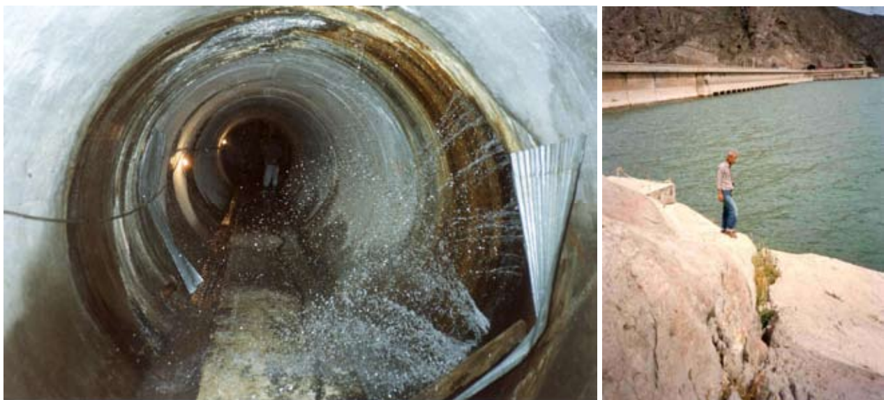
Fig. 10 : Leaking fissure in foundation gallery (left) and trace of fault of Manjil earthquake (right)
