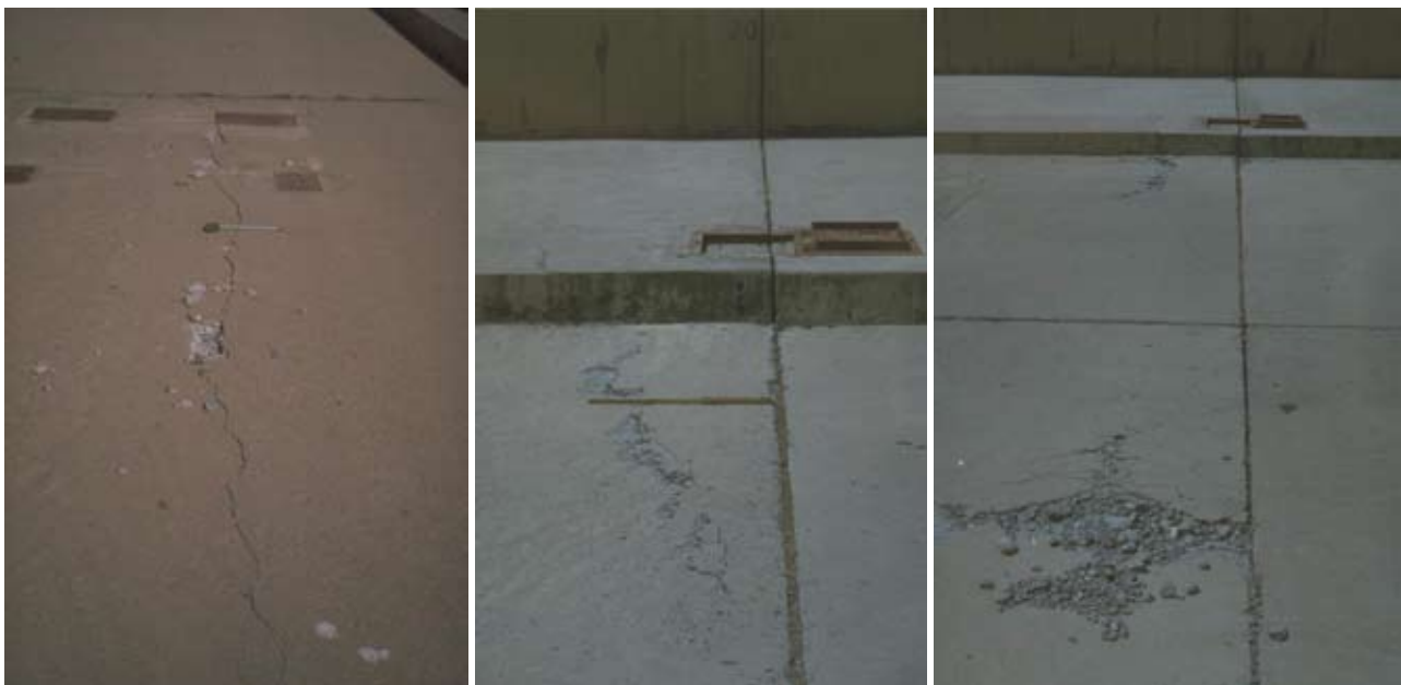
Fig. 5 : Cracks on dam crest due to high compressive stresses: Longitudinal crack (left) and compression shear crack at block joints (centre and right) (Note: Relative movements occurred between some of the block joints)
