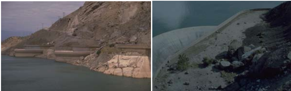
Fig. 7 : Rockfalls at intakes of morning glory spillways on left dam abutment: main rocks could be withheld by horizontal platform above intake (right)
