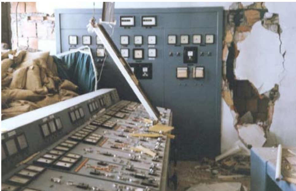
Fig. 12 : Damage in the control room of the hydropower plant caused by ground shaking (Note: The sandbags at the left were placed as protection from missiles as the dam and power plant were attacked by fighter planes during the Iran-Iraq war of 1980-1988)
