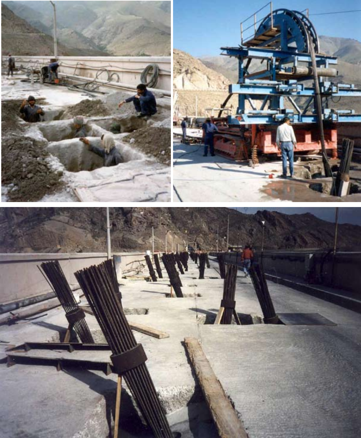
Fig. 17 : Repair work at Sefid Rud dam: Excavation for placement of anchor heads (top left), placement of anchor by homing device mounted on a crawler chassis (top right) and installed rock anchors before stressing (working load of each tendon: 8.4 MN) and final placement of anchor heads (bottom)
