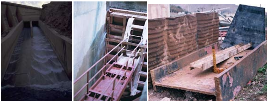
Fig. 8 : Damage of radial gate of intermediate level spillway causing leakage (left and centre) and deformed portion of spillway arm due to high hydrodynamic pressures (centre and right)
