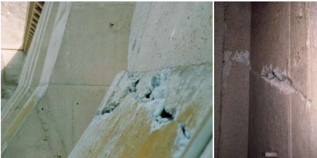
Fig. 3 : Crack at kink location in buttress (left) and horizontal crack along lift joint (right)
