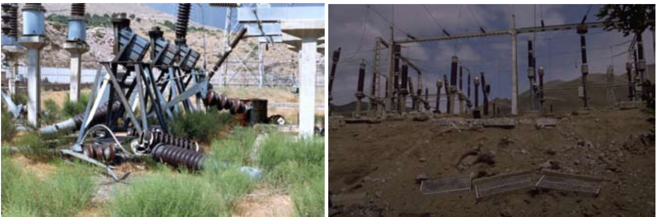
Fig. 14 : Damage of switchyard equipment due to ground shaking and ground movements
