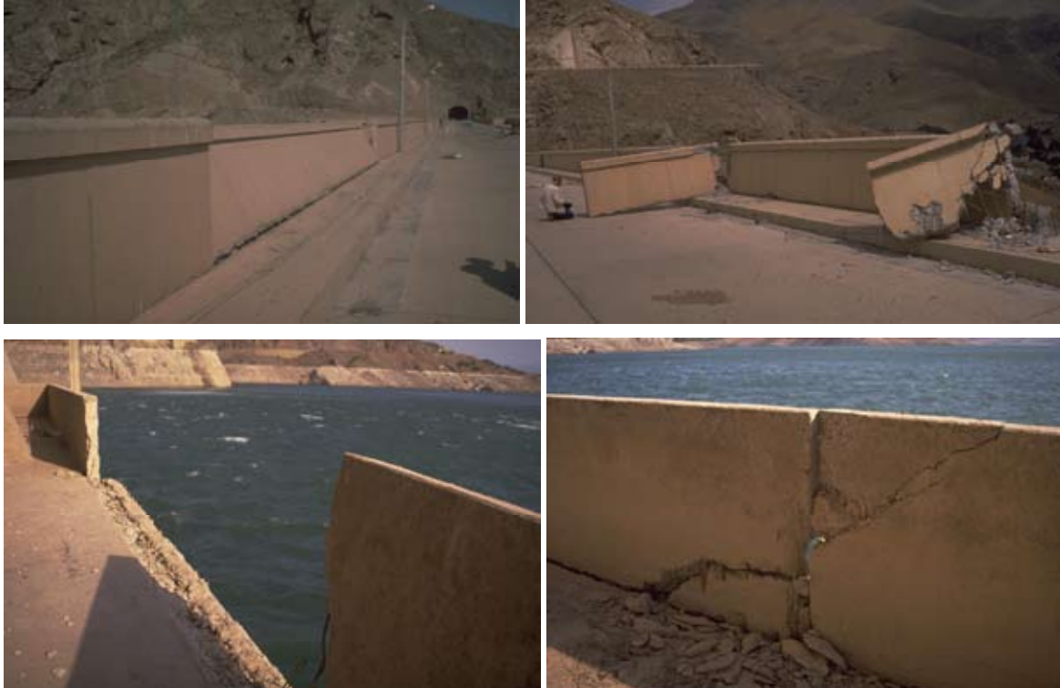
Fig. 6 : Tilting of concrete parapet wall on downstream crest (top left) and secured tilted wall after the earthquake to protect it from falling on the powerhouse (top right), damage at upstream face parapet walls above intake gates (bottom left and right)
