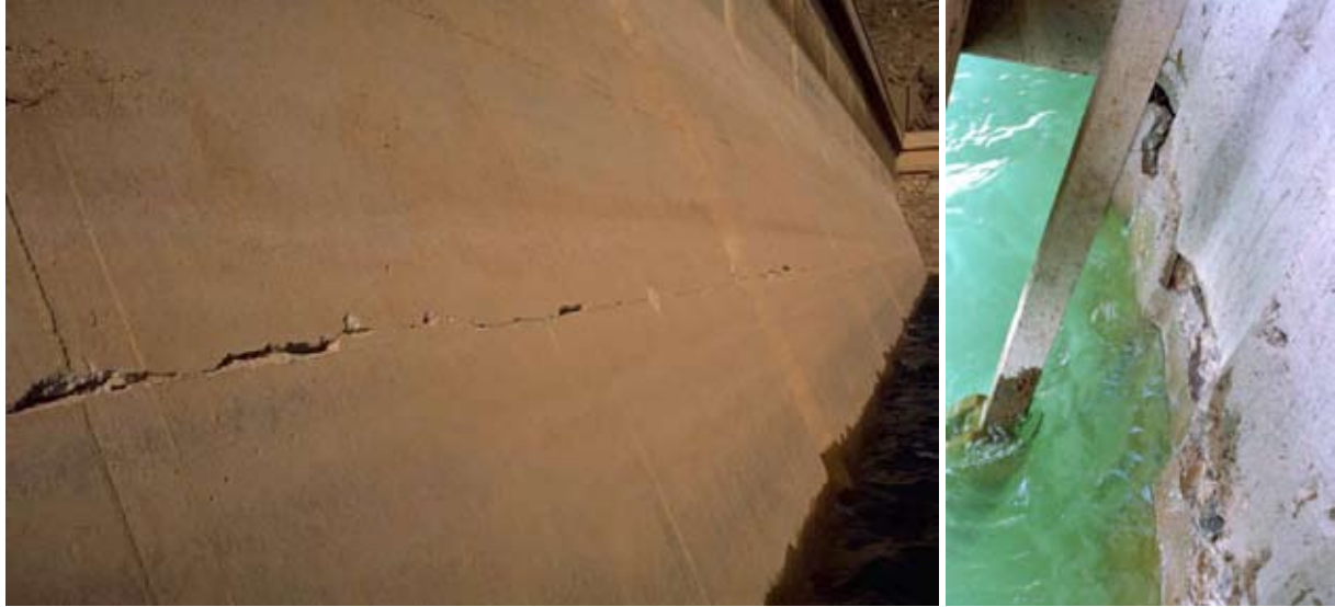
Fig. 4 : Horizontal crack at upstream dam face through several buttresses along lift joint (left) and horizontal crack and spalling of concrete above intake gates (right)
